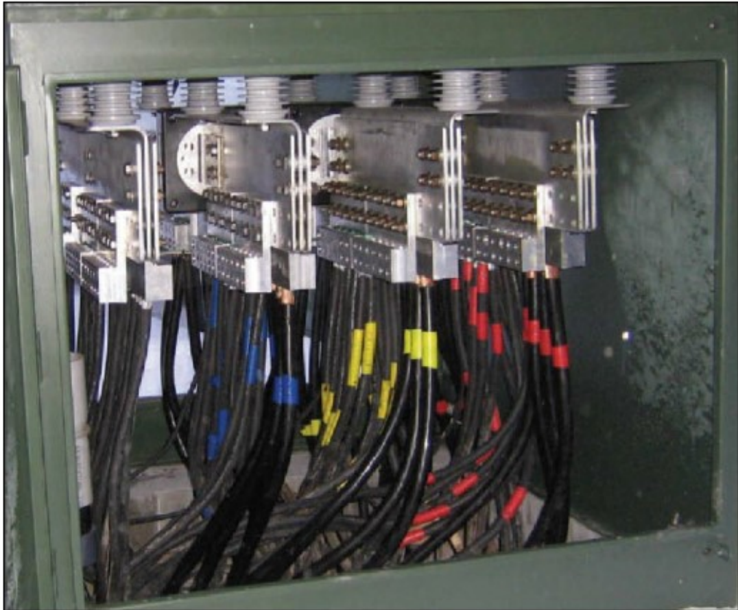
LOAD SIDE CONNECTIONS
