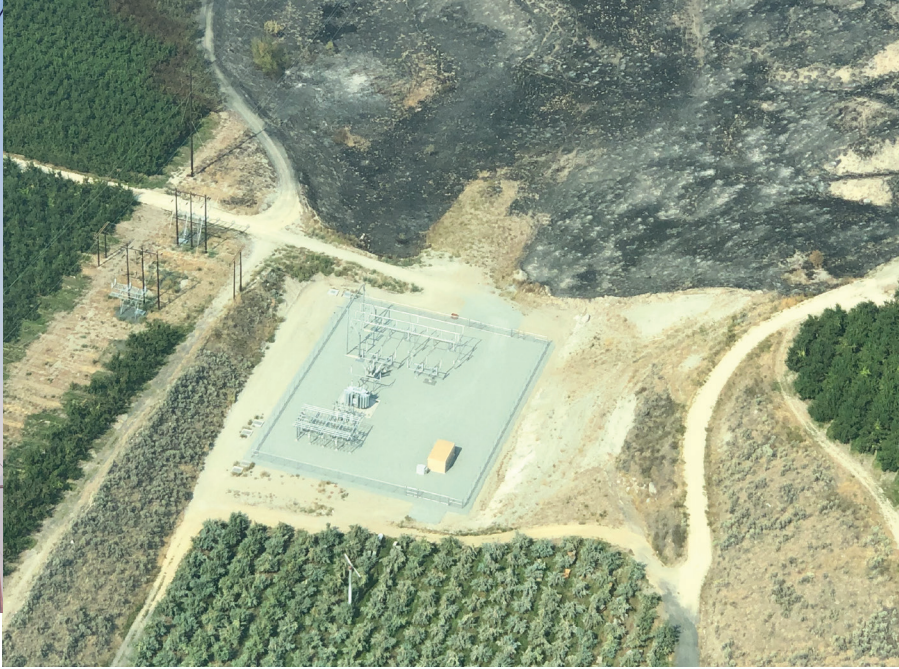
(From left) The Foster Creek transmission line presented several challenges for rebuilding on a hillside. Large structures broke apart in multiple places along multiple lines. Fire nearly reached the new Chicken Creek substation.
